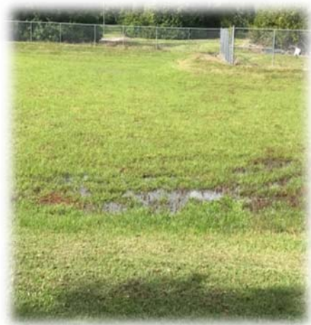
Figure 9 - Ponding in Rear of the Facility on January 24, 2020
