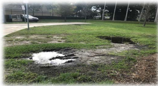
Figure 10 - Permanently ponding water in grassy area on February 19, 2020
