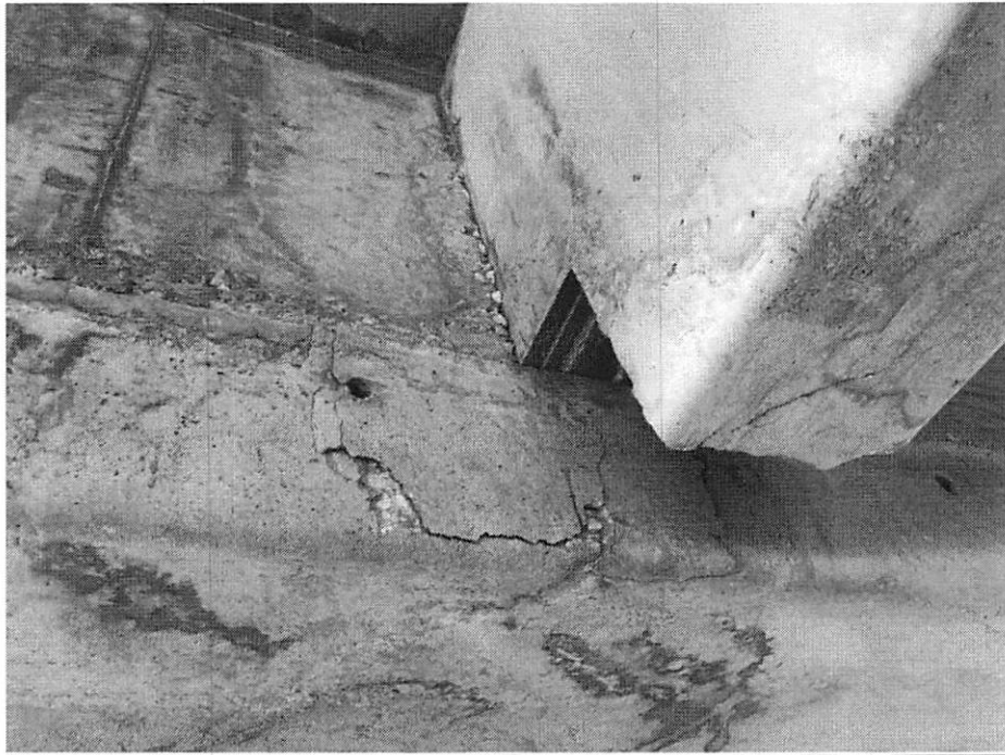
Exhibit 15: Spalling and Cracking on a soffit beam at a joist support.
