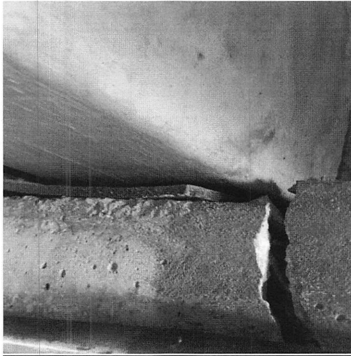
Exhibit 11: Loose bearing pad. Joist is not bearing on the front half of the cracked haunch.
