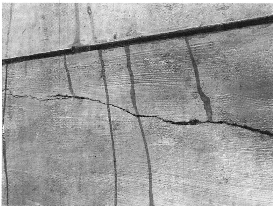
Exhibit 18: Slab cracks along the sides of a soffit beam.
