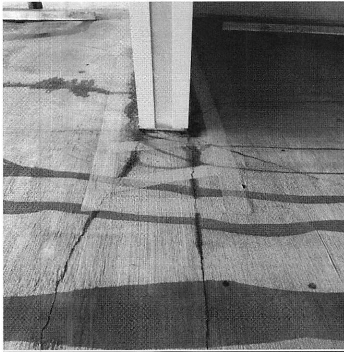
Exhibit 20: Slab cracks along the sides of a soffit beam.
