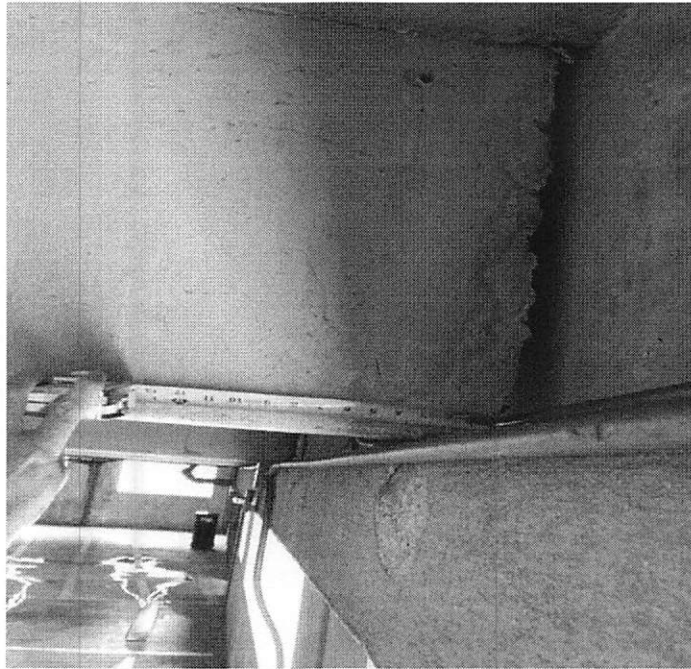
Exhibit 14: Spalled face of a haunch below a supported joist.
