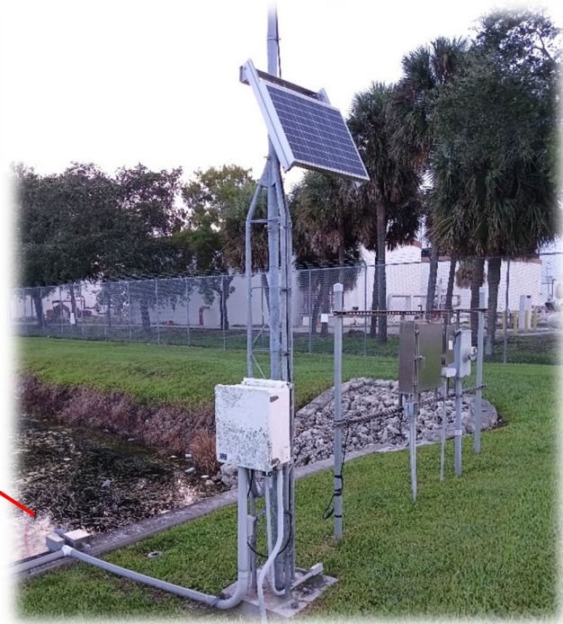
Water Level Monitoring Device
