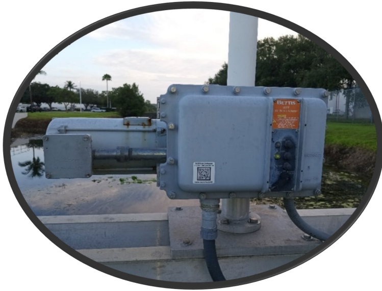
Water Control Gate Motor
